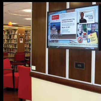
Video Switching and Distribution
